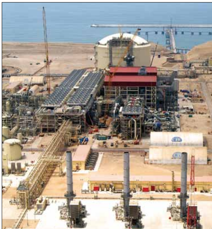
The liquefaction plant is on the Pacific coast at Pampa Melchorita.
